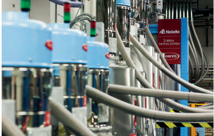
Northern Europe's most modern materials handling system ensure quality and productivity.
