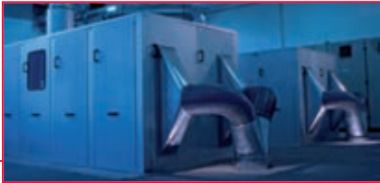
Sludge treatment plant | Italy
